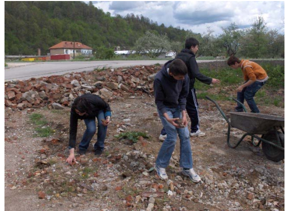
Children in Bosnia – Herzegovina removing the remains of an old electricity station
